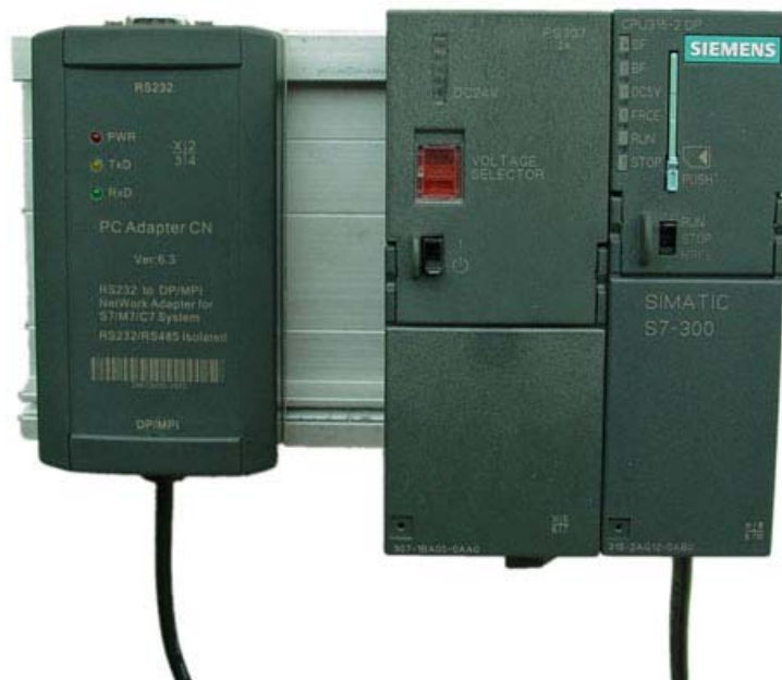
PC Adapter CN has been installed on the S7-300PLC rail
